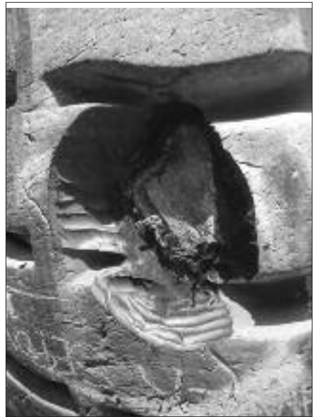
Fig 24. Deep tread rock cut – If left unattended will cause tread rock cut separation.
